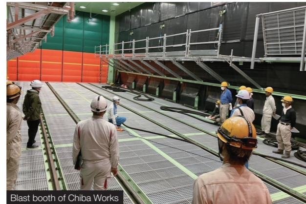
Blast booth of Chiba Works
