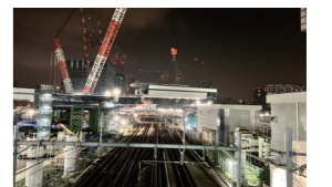
New construction of crossing section of Kanryo 4 Expressway within Shinagawa Station building
