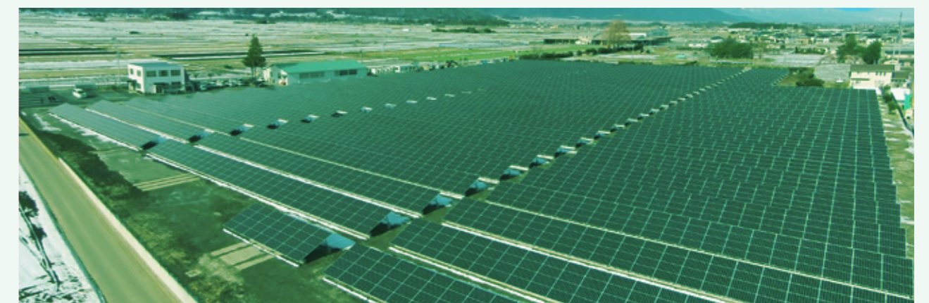
Matsumoto Power Plant
